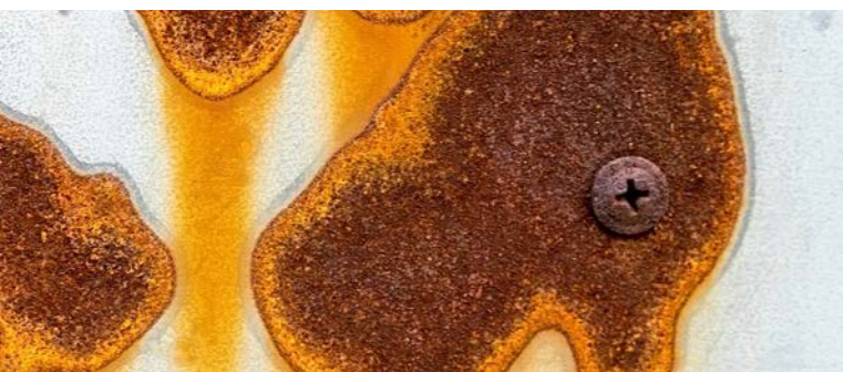
Fig 2.3 Galvanic Corrosion of Aluminium Cladding Sheets in contact with Stainless Steel Screws
