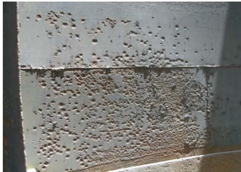
Figure 2.1 Pitting corrosion occurring on thickener tank under a biofilm layer
