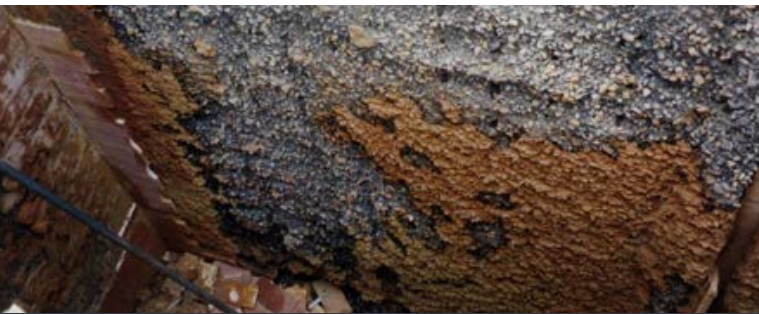
Fig 2.5 Biogenic corrosion in enclosed head space of concrete bar screen chamber
