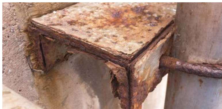
Fig 2.4 Biogenic corrosion of pipe brace/support in wet well
