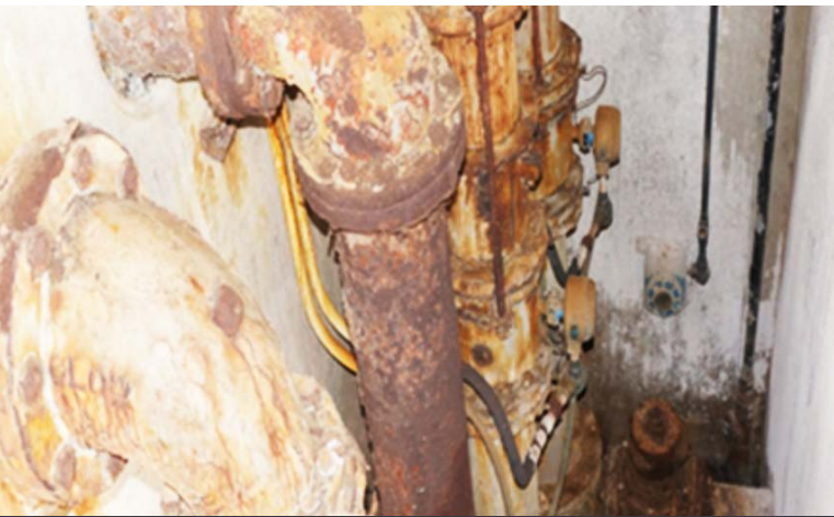
Fig 2.2 Graphitic Corrosion on Primary Intake Pipes
