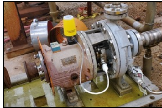
Chesterton Connect installed on the pump.
