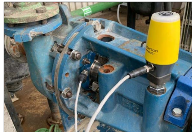
1510 installed with Chesterton Connect monitor
