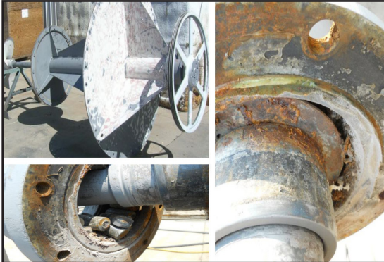
Greasing hard to seal shaft bearings was unreliable. Annual failure was expensive.
