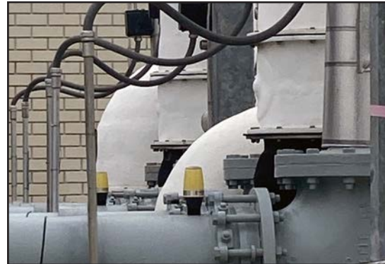
Submersible pumps with Chesterton Connect Sensors.
