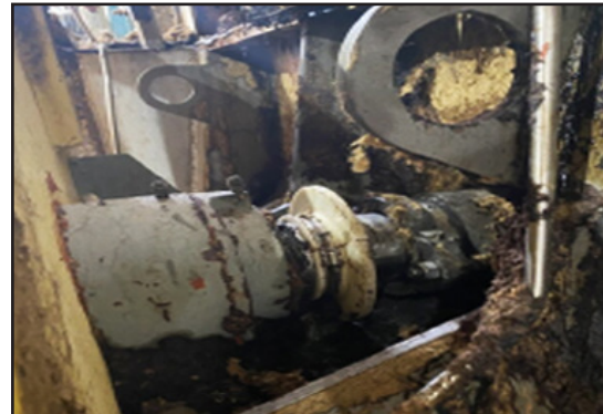
Equipment before AMPS unit installation. It was very difficult to access bolts to make any adjustment, and unsafe to do while running.
