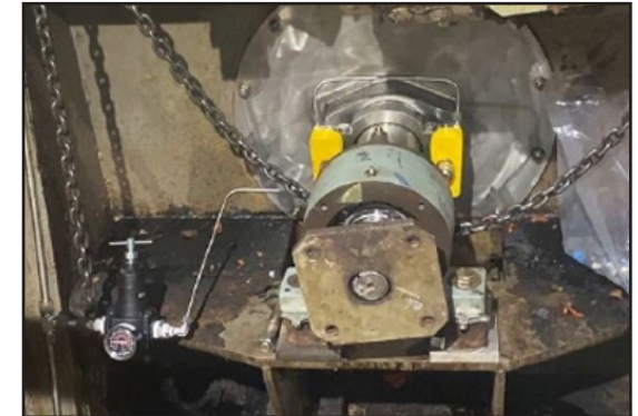
Equipment with AMPS units installed on both bolts, enabling constant, even loading and offering the ability to safely make adjustments.
