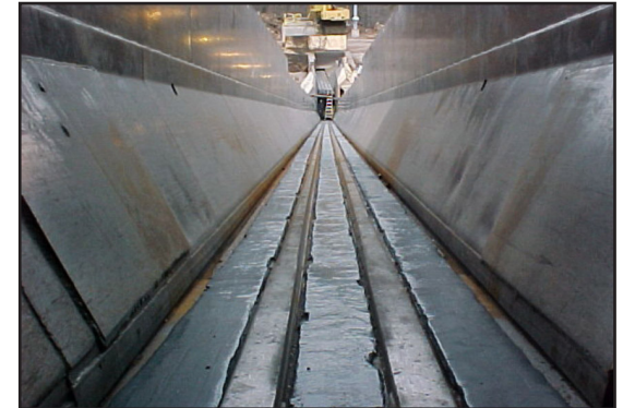
Chute protected with ARC BX1*
