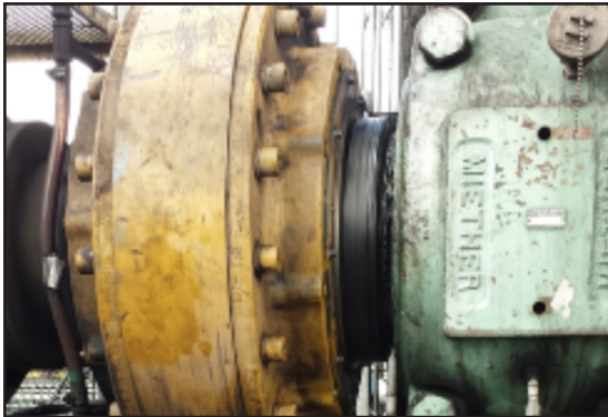
The plant's conveyor equipment leaked excessively.
