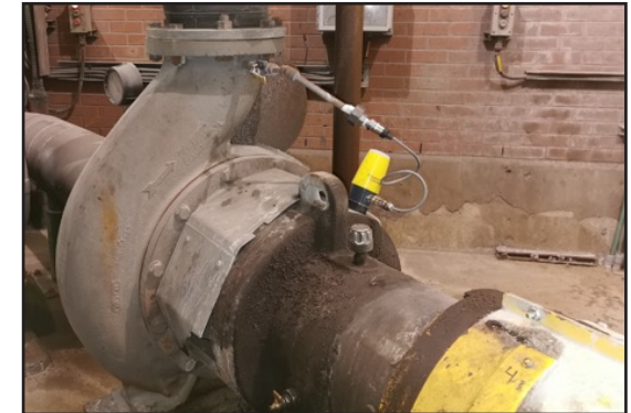
Chesterton Connect™ sensor installed and operating.
