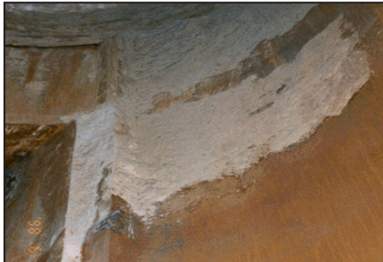
Severe corrosion inside the stack
