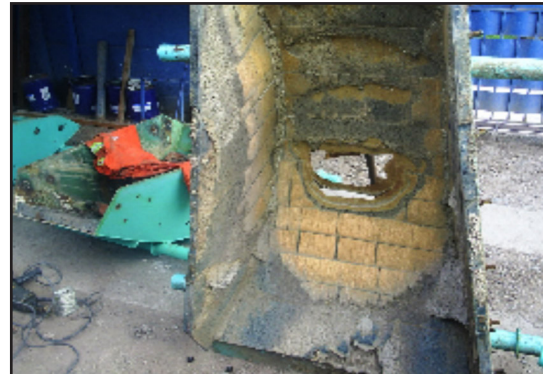
Rubber and tile lined chute after 1,500 hours
