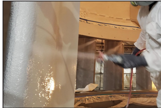
Plural component spraying of ARC S1HB up to 150 mils in a single coat.
