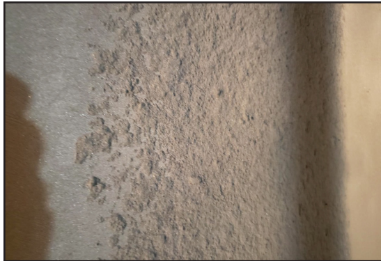
Damage to wicket gates.
