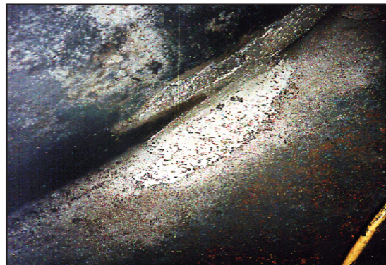
Cavitation damage is evident after proper surface cleaning
